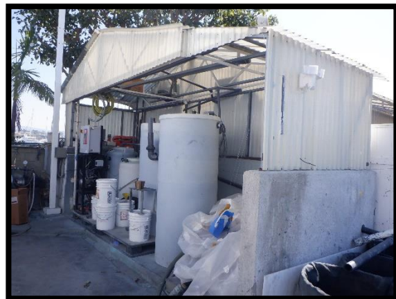
Water Treatment Area
