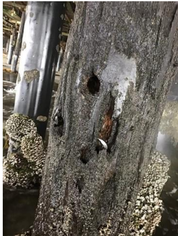
Photo 4-11: ZONE 1 - Timber Pile Moderate Defect, Pile 47c
