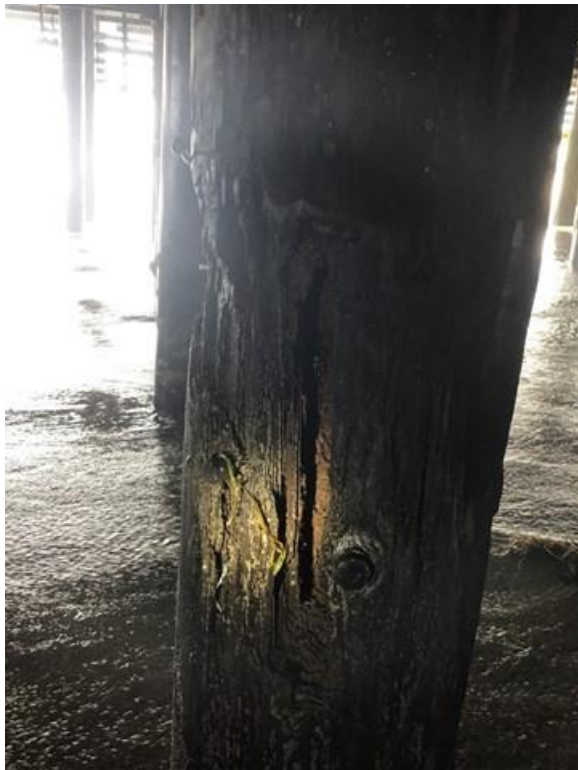
Photo 4-10: ZONE 1 - Timber Pile Major Defect, Pile 46f
