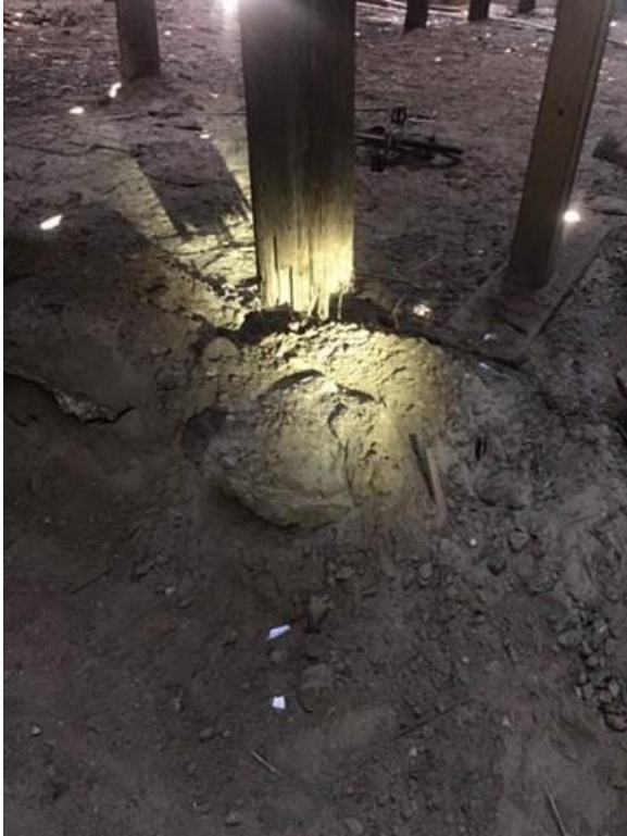
Photo 4-8: ZONE 1 - Timber Pile Severe Defect, Pile 11.5q
