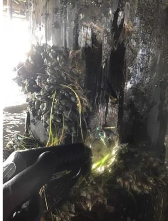
Photo 4-9: ZONE 1 - Timber Pile Severe Defect, Pile 47i.7
