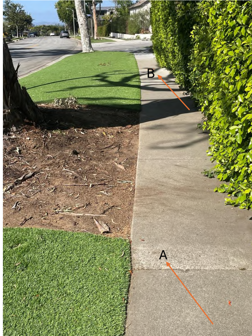
Proximity of sidewalk lifting (A) and replacement (B)
