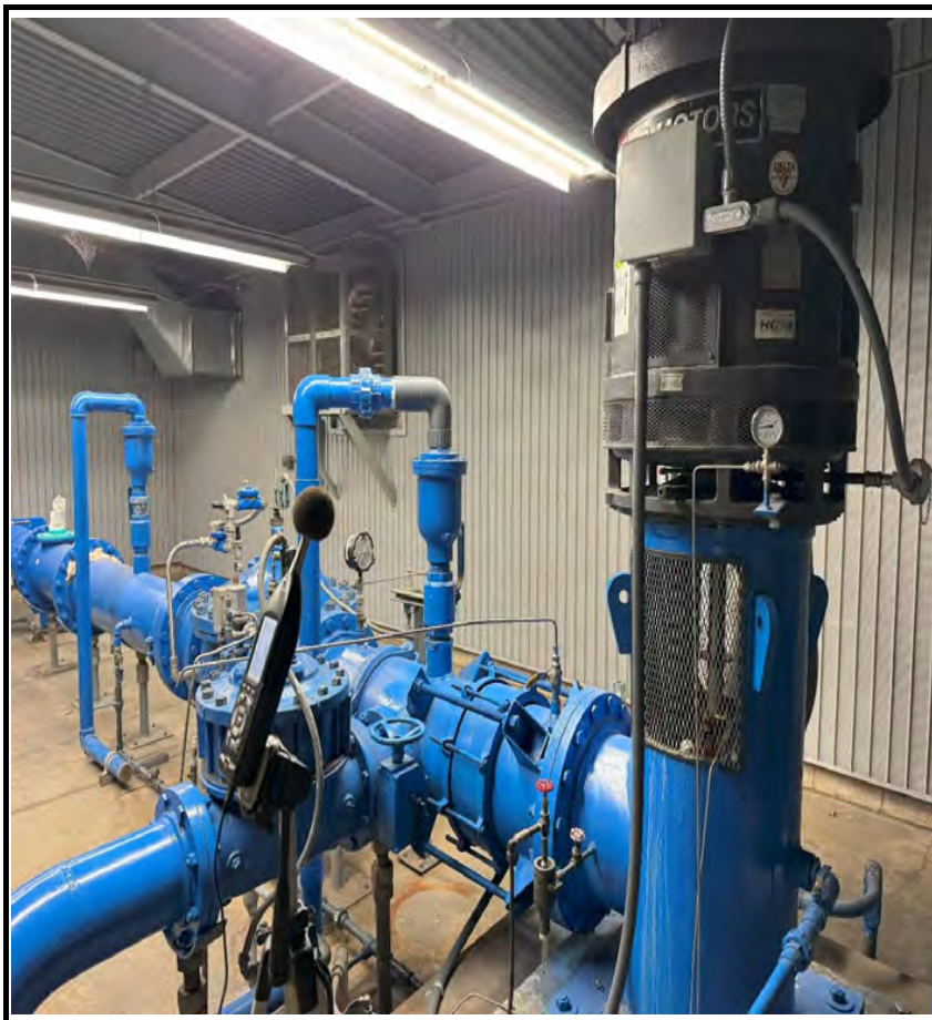
STNM interior looking SW, active water pump on the right, active interior air extractor fan on the left ( on western wall ).
