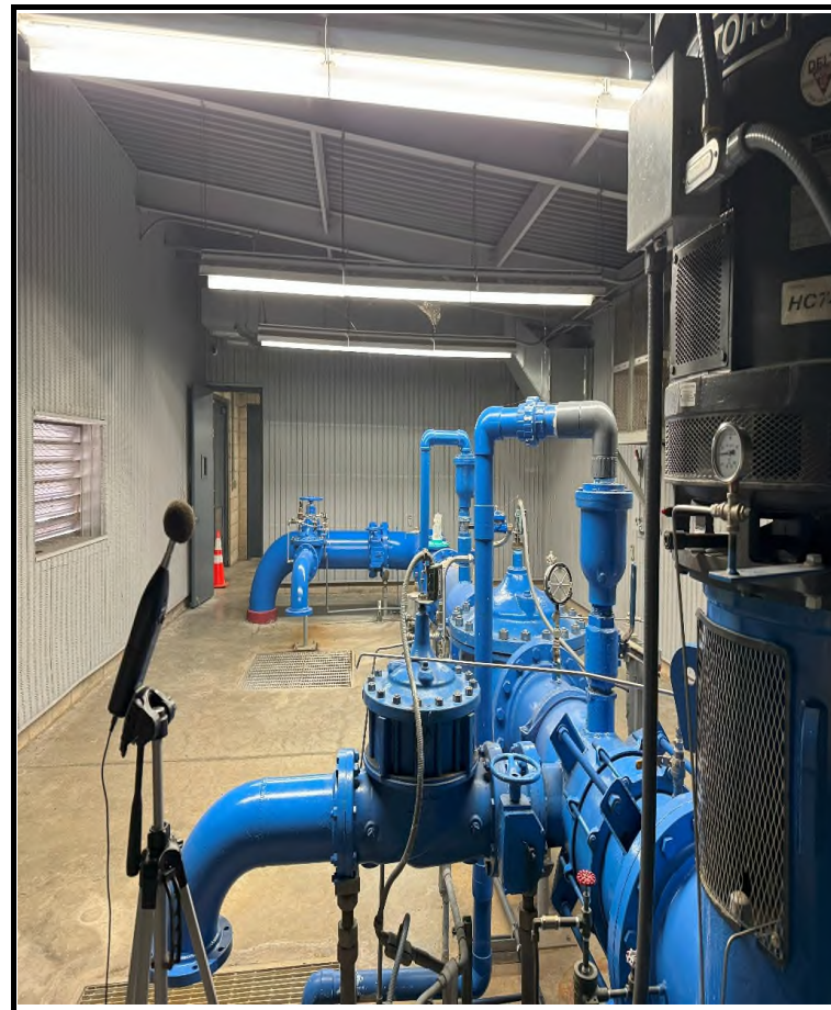
STNM interior looking S from northern water pump towards control room ( through open door in southern wall ). Pump continually in operation. Air extractor fan on western wall also on, making significant noise.
