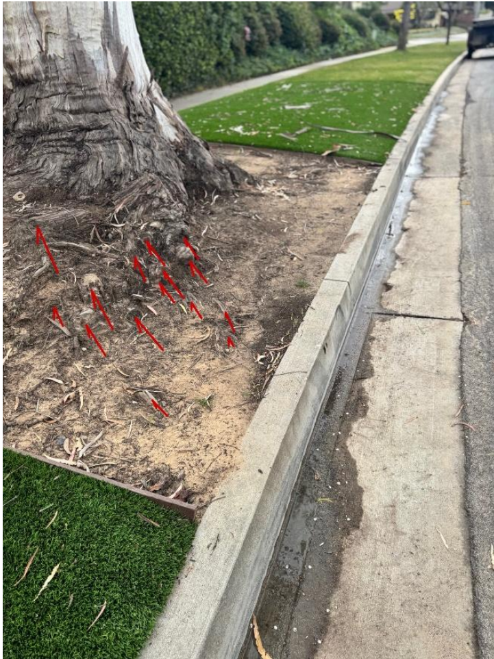
PHOTO #1 – ARROWS INDICATE CUT ROOTS
