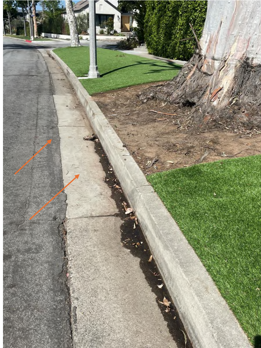
View of repair gutter and asphalt street in proximity to Tree ID 972864
